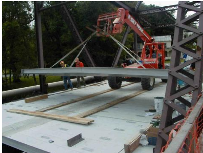
Figure 17 Photo showing the installation of an FRP deck panel for deck replacement project in New York State (courtesy NYSDOT and FHWA).
