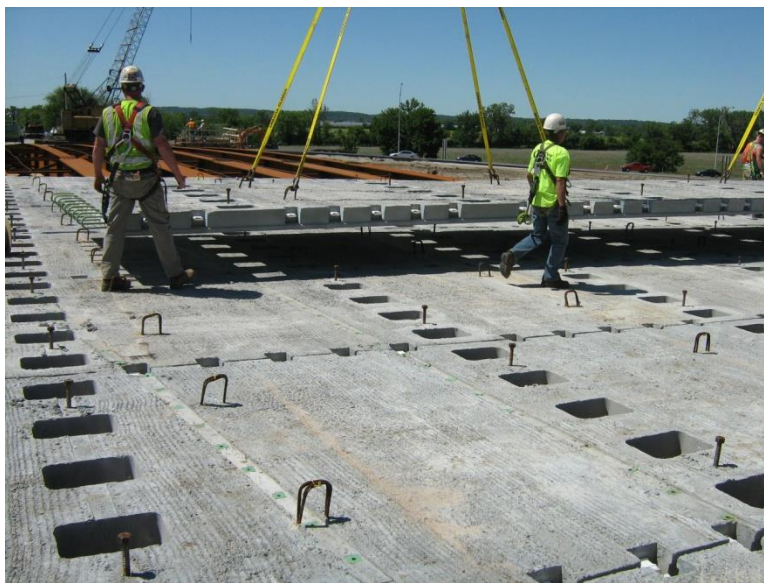
Figure 1 Bridge deck being constructed with full depth precast concrete deck panels (courtesy Iowa DOT).
