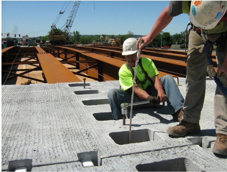
Figure 2 Construction workers adjusting the elevation of the full depth precast concrete deck panels by adjusting leveling bolts (courtesy Iowa DOT).
